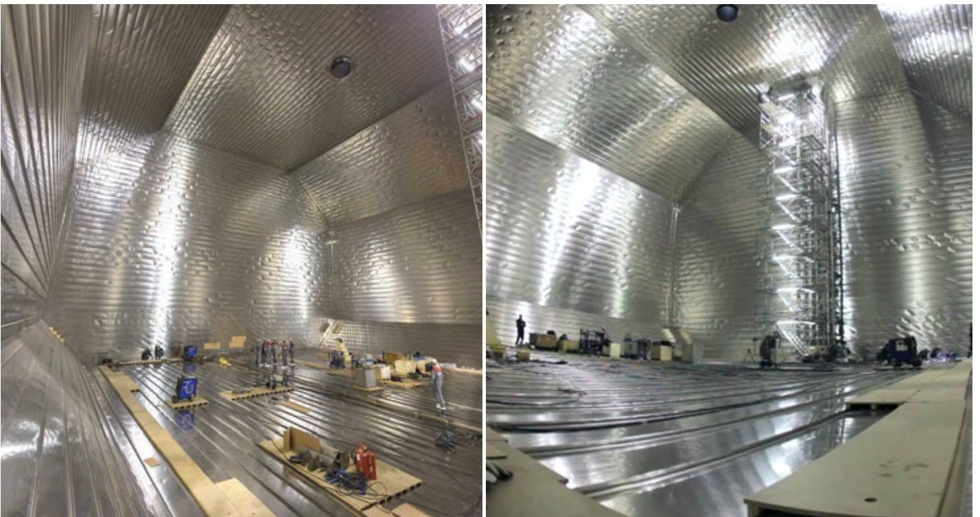
Testing and Repair of Membrane Containment Systems - The 1st total replacement of LNG membrane containment system in Asia
