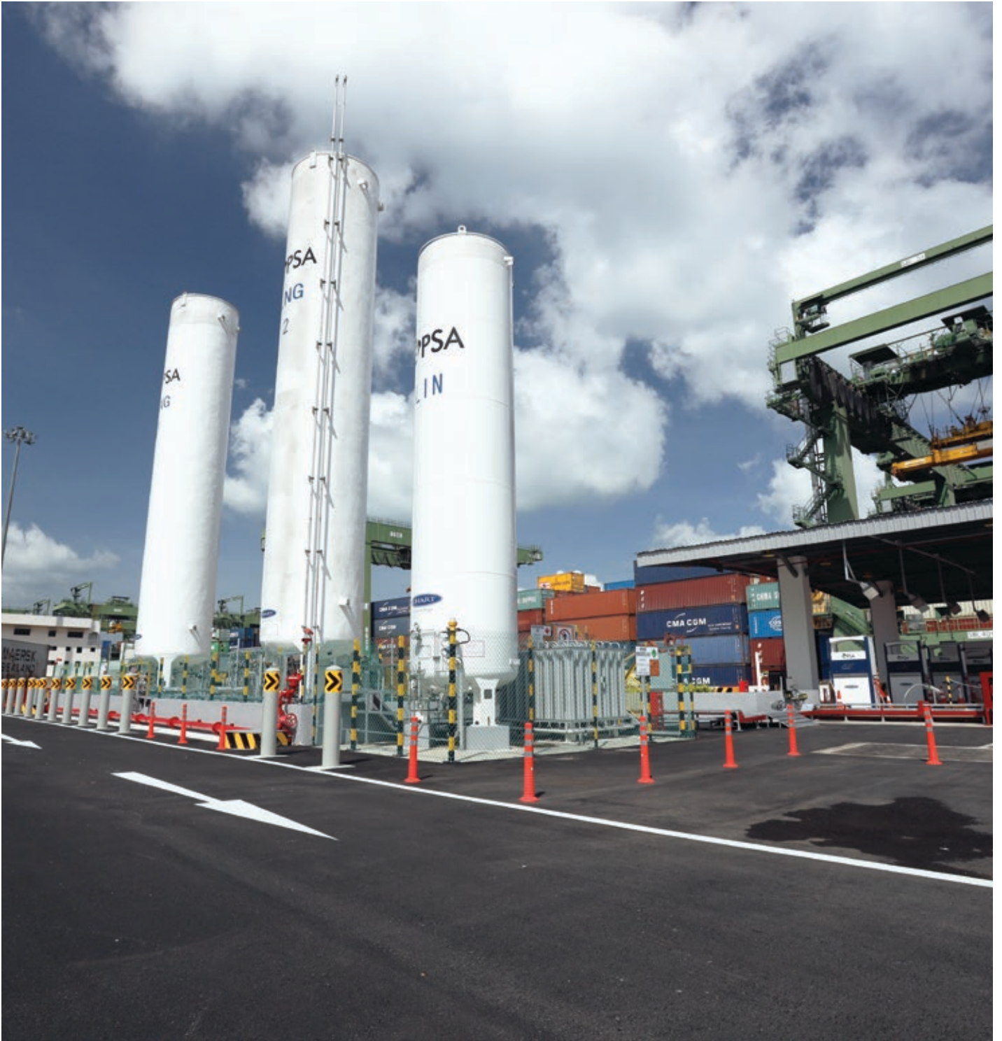
Engineering, Procurement, Construction and Commissioning (EPCC) solutions - The 1st LNG storage and refuelling station in Singapore
