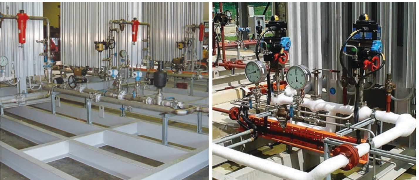
Commissioning of automated vaporization system
